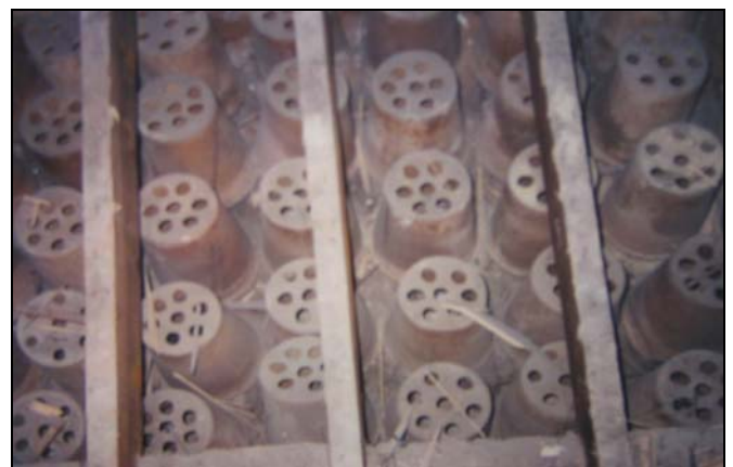
Figure 7. Air chamber with the clay vessels, under the orchestra pit (1989 picture [3])
